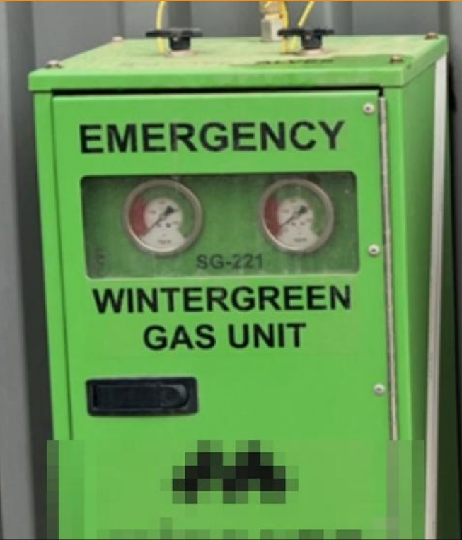
EMERGENCY GAS SYSTEMS Underground emergency notification and response infrastructure.
