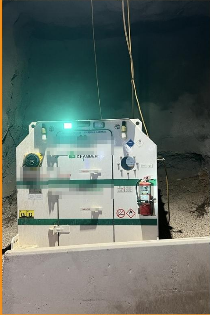
UNDERGROUND REFUGE & EMERGENCY SYSTEMS Critical life-safety systems supporting underground emergency readiness and operational resilience.
